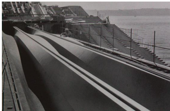
Figure 1. Formworks for concourse beams under preparation. "Viking ships upside down." Photo by Max Dupain [pending permission, (taken from Yuzo (2001) p.50)].
